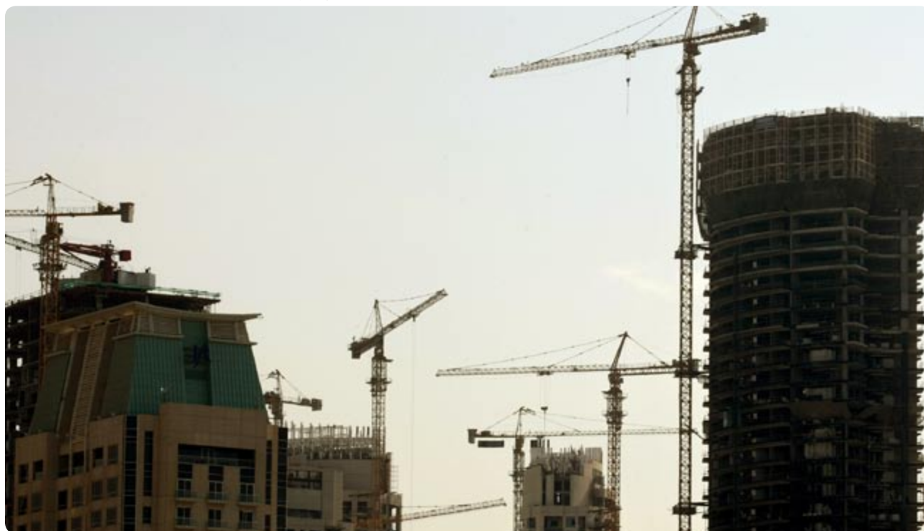
Cranes are erected at the Dubai Marina, where scores of skyscrapers and towers are under construction
