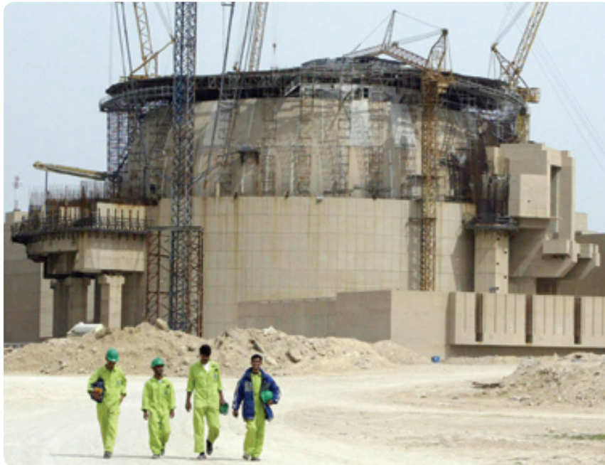
Iran's Bushehr nuclear reactor is expected to become operational by July 2007
